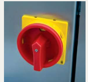
The main circuit breaker
