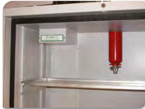
Fire-extinguisher installed in a safety cabinet
